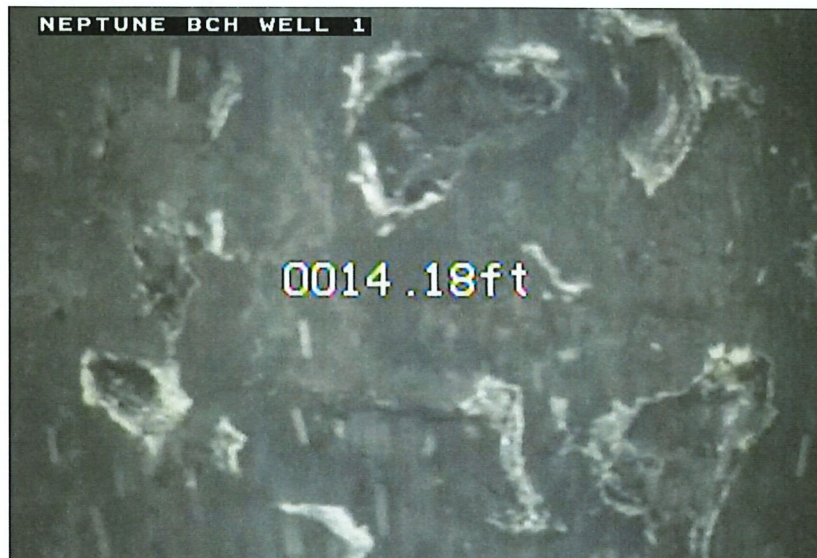
Photograph 1 Typical Casing Pitting
