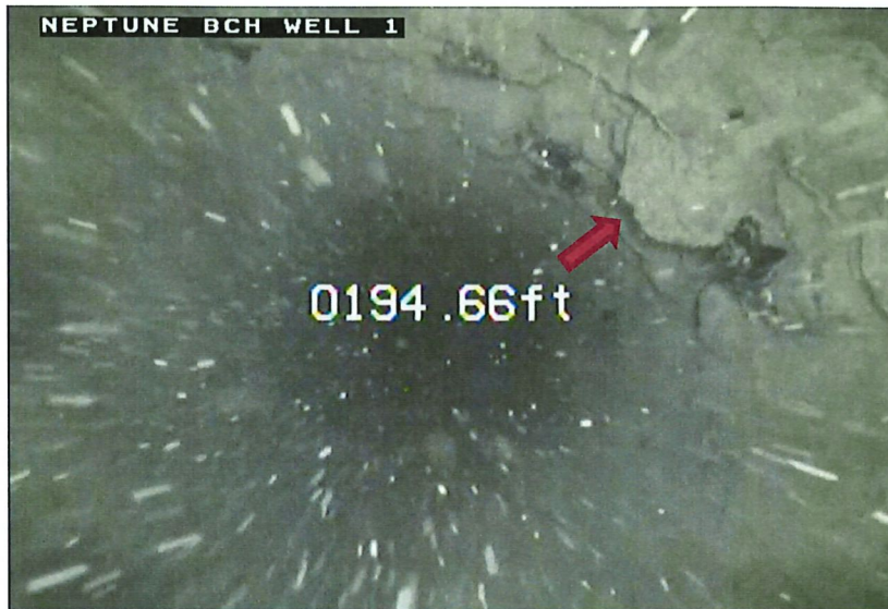
Photograph 3 - Casing Incrustations (Looking Down in to Well)
