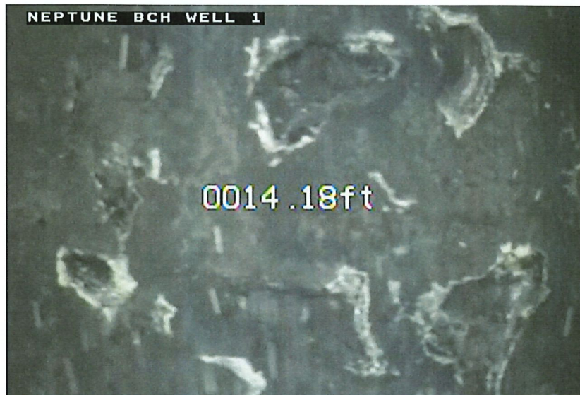
Photograph 1 Typical Casing Pitting
