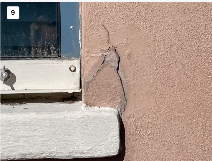
Cracking stucco at window frame
