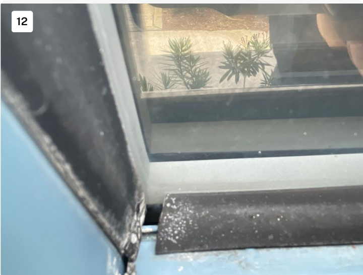
Openings at window seal corners
