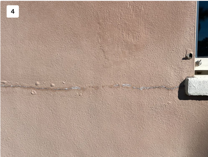
Cracking stucco and bubbling paint
