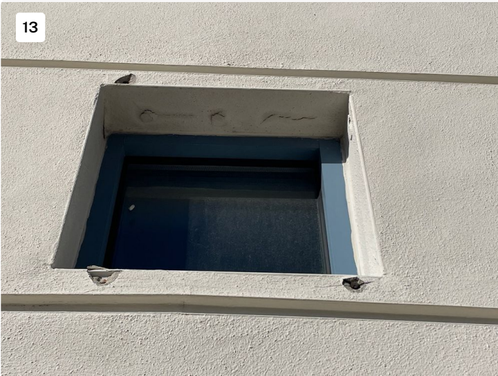
Cracking stucco around windows
