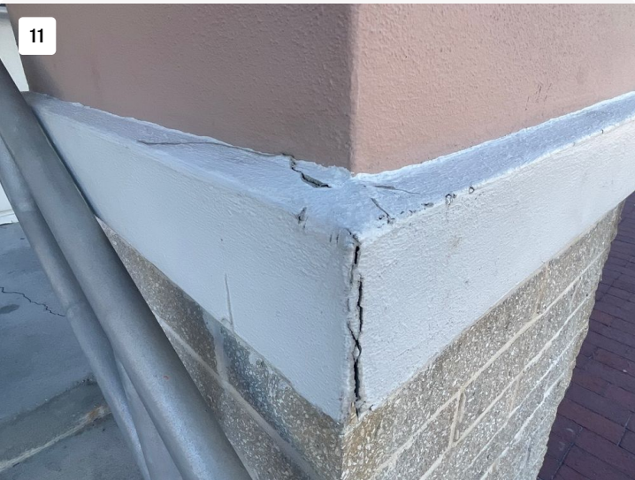
Cracking at pillars
