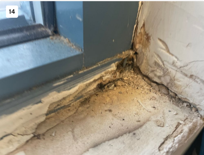
Interior window sill damage
