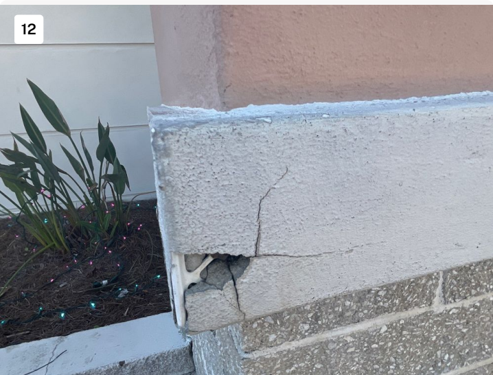
Cracking at pillars
