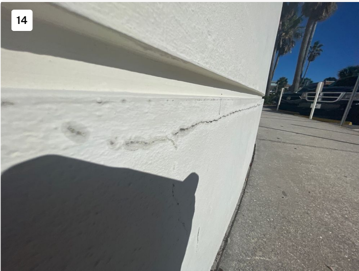
hairline cracking in stucco
