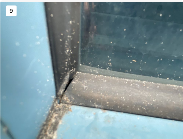
Openings at window seal corners
