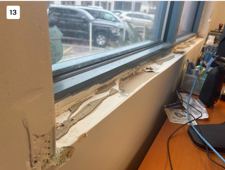
Interior window sill damage
