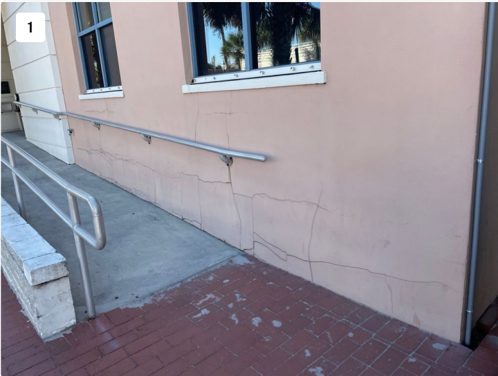
Major stucco damage
