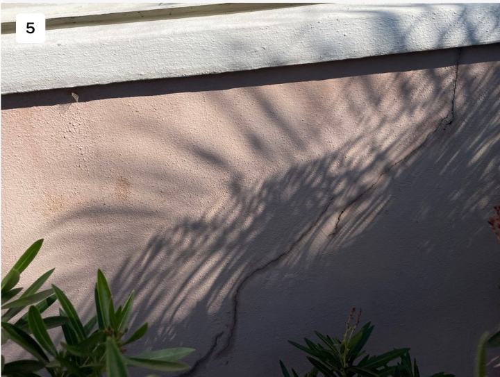
Cracking stucco below windows
