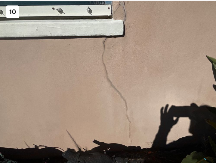
Cracking below window frame
