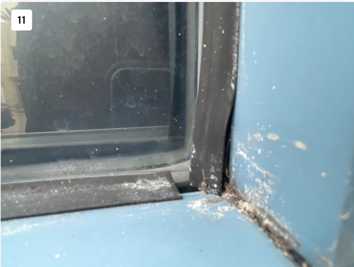
Openings at window seal corners
