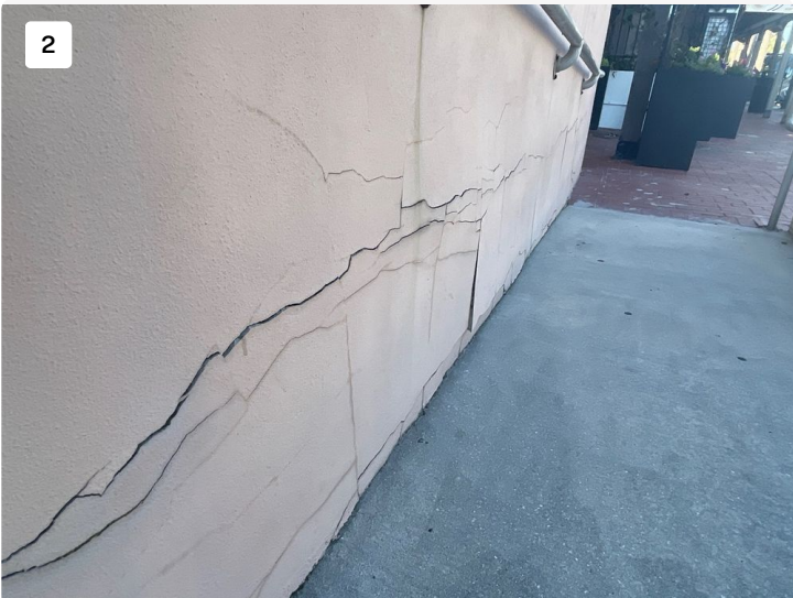
Handicap ramp stucco damage
