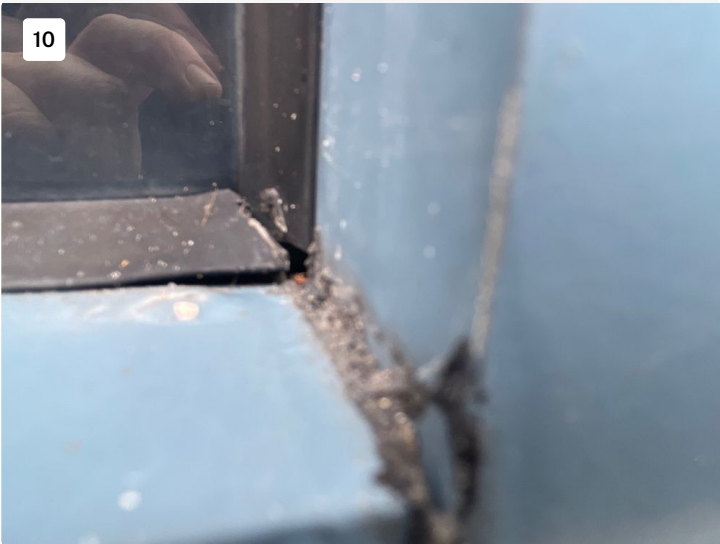
Openings at window seal corners
