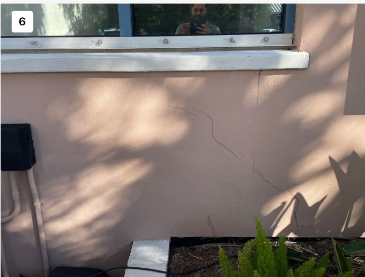
Cracking stucco below windows
