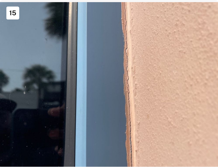
Window perimeter sealant cracking
