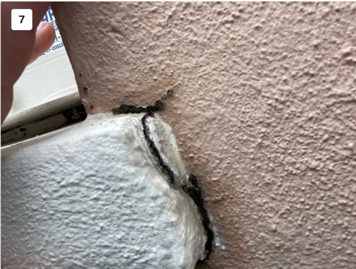
Stucco cracking at window frame
